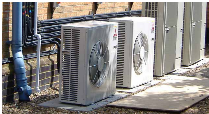
Example air source heat pump compressors.
