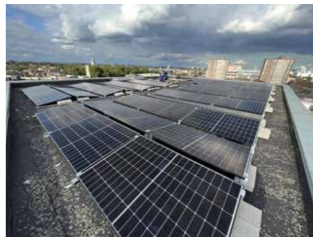
Example PV Panels.
